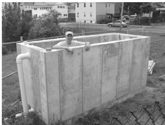
Figure 1. A pre-cast concrete structure was constructed for the wood filter field experiment in Providence, Rhode Island. The filter's inside dimensions were 1.4*1.2*3.3 m (H*W*L) - equivalent to about 5 m 3 volume. The filter was outfitted with 27 wood filter modules containing about 115 kg of (dry) shredded aspen wood.
