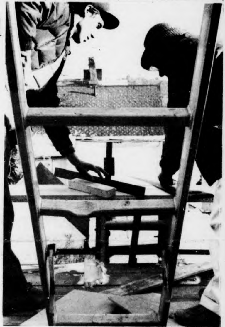
Construction workers continue on renovation of new house while oil clean-up continues four stories below. (See page 15 for further details on new house.)
