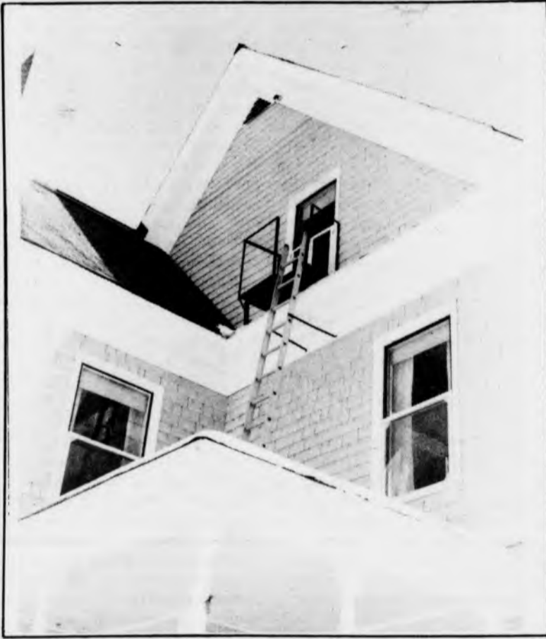
One of the visible violations cited by Inspector Baillargeon. (Ooi)
