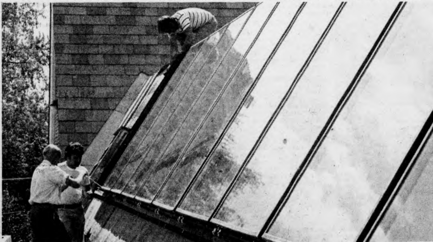
Workmen install new solar panels atop Chase Hall. Work remains to be done installing other equipment before solar heating and water heating facilities are completed.
